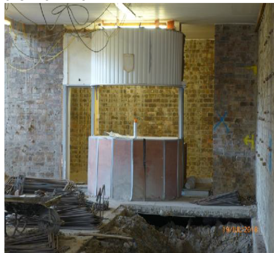
Lower GF – Section of Protection to the Reception Desk has come away, no works ongoing at this area at present
